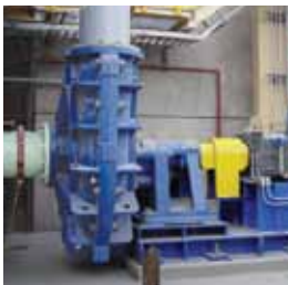
Left: A large copper gold installation in Argentina has upgraded their existing 450mm pumps to the latest 450 MCR design
