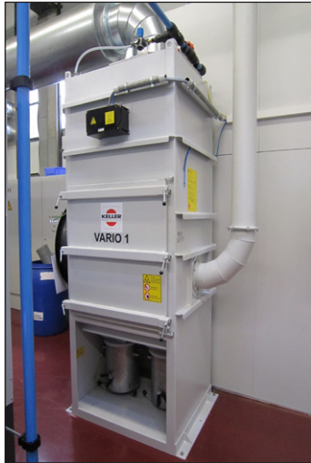
VARIO 1 eco as a central vacuum system
