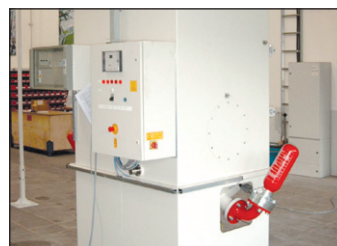
Explosion suppression by automatic entry of extinguishing agent
