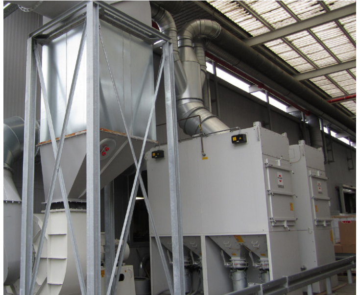
Two VARIO 6 eco units with a total air flow of 40.000 m 3 /h condition the exhaust air following combustion with a renewable thermal oxidation process
