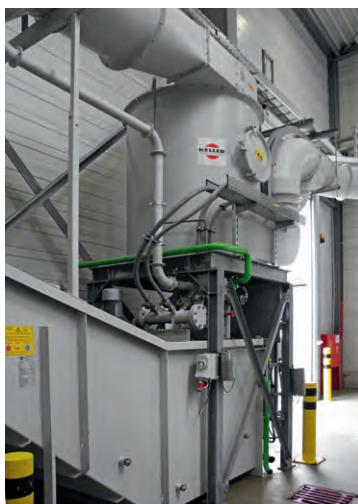
Wet scrubber with water treatment tank
