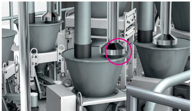
Dust separation with collection hoods at the weighing scales above hoppers.
