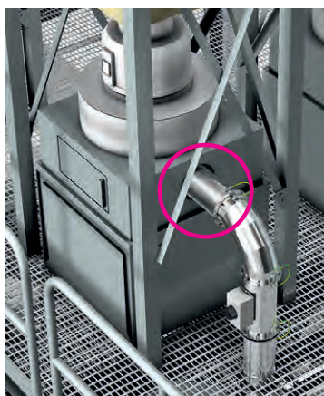
Closed extraction to separate the bulk material during the feeding of raw material (Big Bags or sacks)
