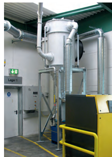
Central vacuum suction system
